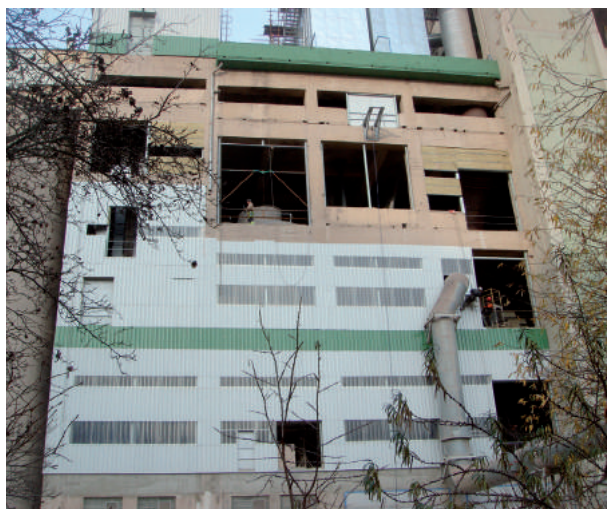
Significant reduction of noisiness was achieved by jacketing the raw material mill
