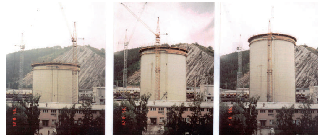
Construction of the clinker silo – the pictures always taken after one week
