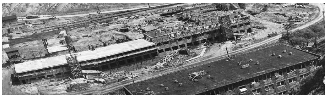
Construction of the new cement plant – sanitary facilities, workshops and the AB building in the front
